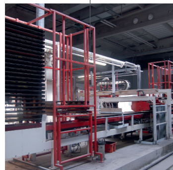
26 Flat depositing device-dry side
