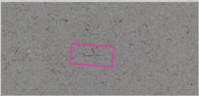
Bounding box pink: Crack
